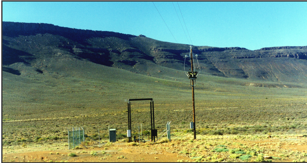
Figure B.19: Injection and abstraction boreholes in Calvinia
